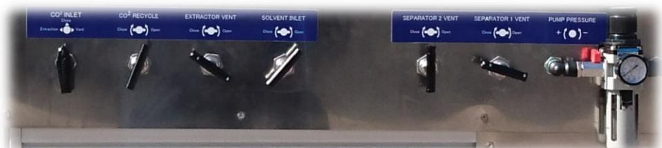
Fluidic control panel with valves for system filling, venting the vessels, recycling, pump pressure control
