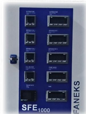
Electronics control panel
